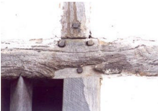
Figure 8. An RBT mortise repair to a rail. New timber is set back behind the retained historic surface.
