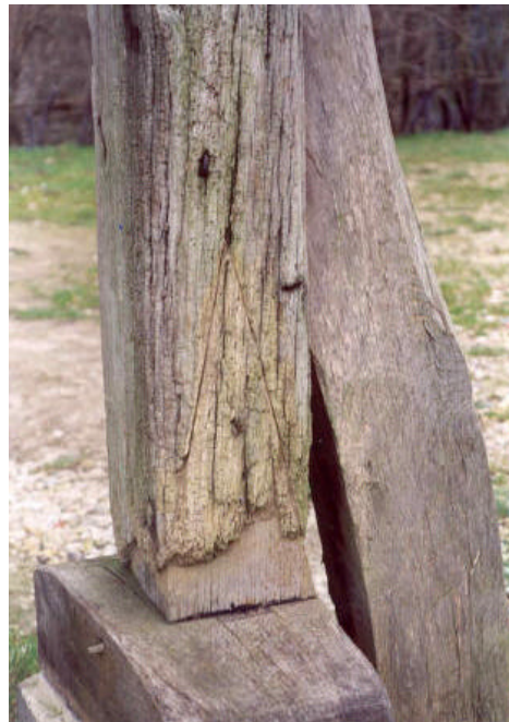
Figure 9. An RBT V-scarf repair with surface veneer reapplied. The perpendicular cuts by circular or band saw are just visible.
