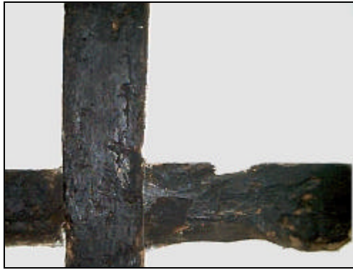
a. Decayed rail with failed tenon.
